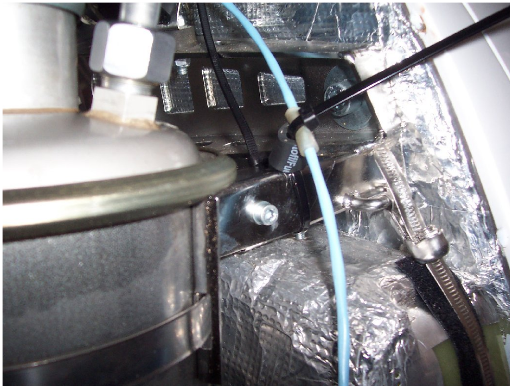
Access to right centre mountings behind oil tank
