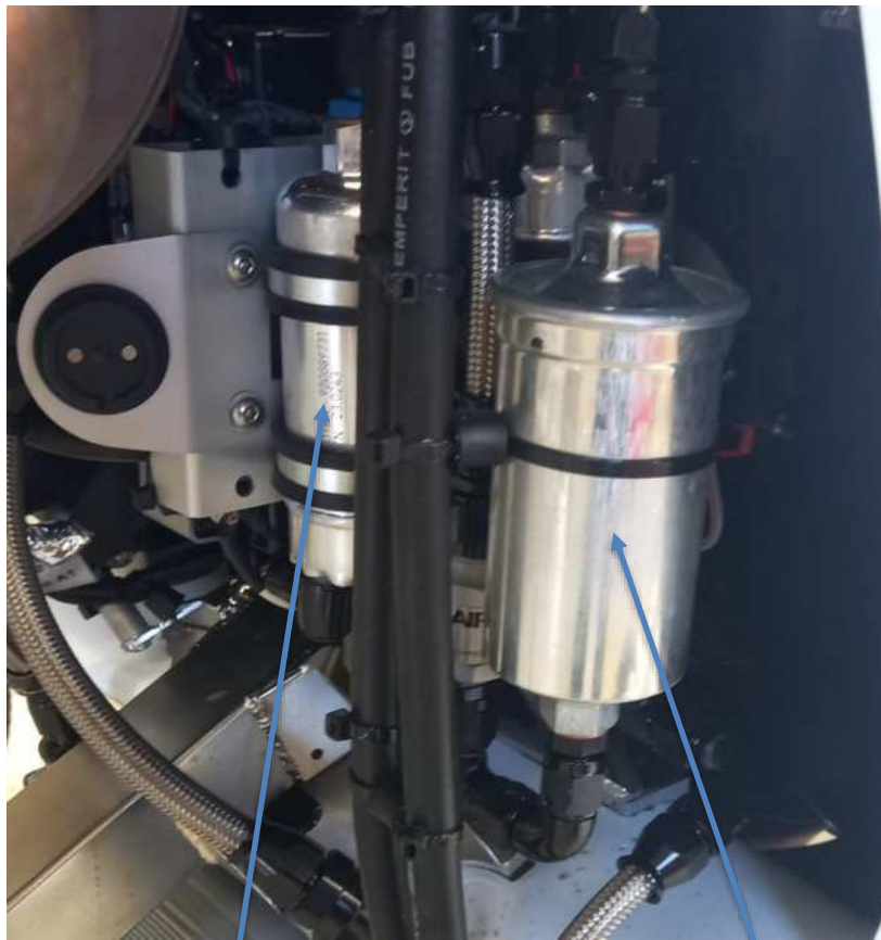
Figure 2 - Location of fuel pumps (within this box) and quick-change fuel filter (916 engine)
