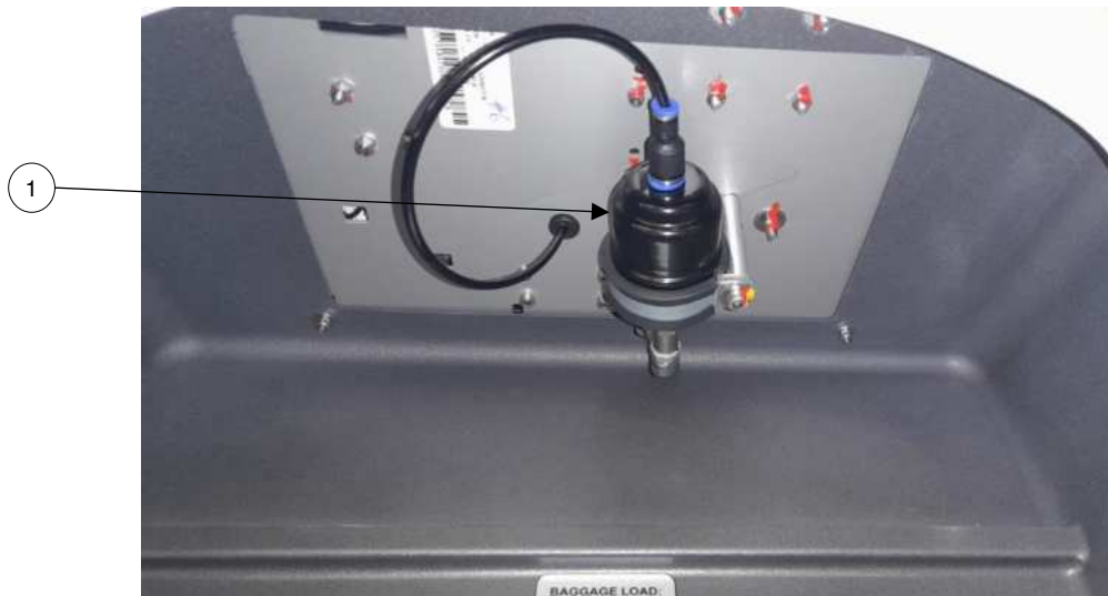
Figure 2 - Location of Filter / Dryer
