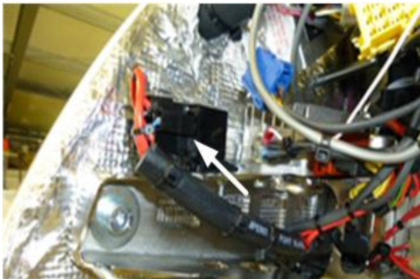
Fig. 3 – Mounted main relay
