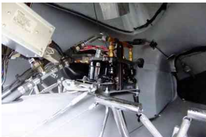
Electrically driven compressor
