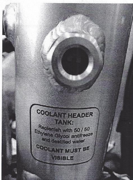
Photo of viewing window, with meniscus of coolant showing.
