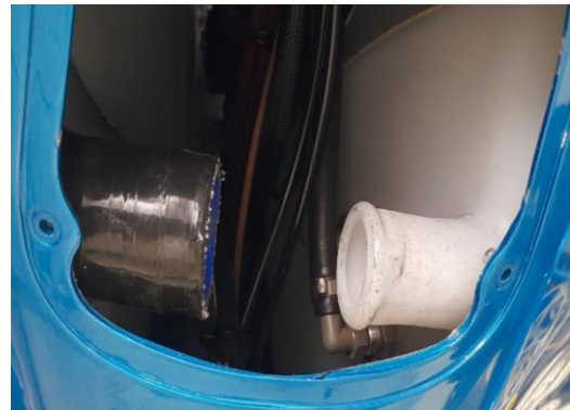
Figure 15: fuel tank connection removed
