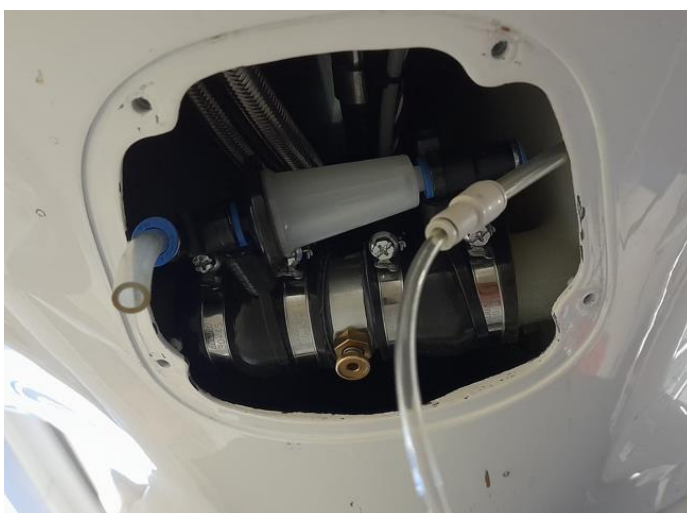
Figure 34: Disconnected vent hose from filter and pressure test device connected to vent line
